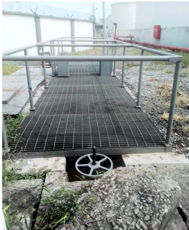
Oil water separator system
